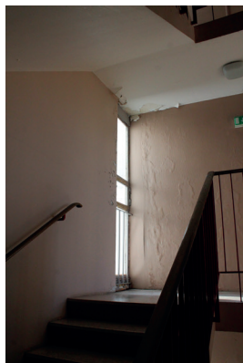
Infiltrations ; circulation verticale principale
